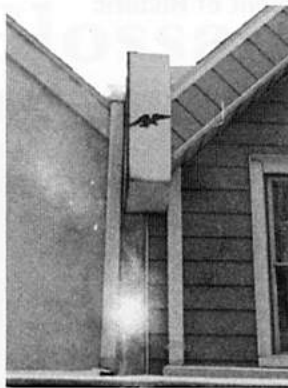
Inappropriate gutter treatment
