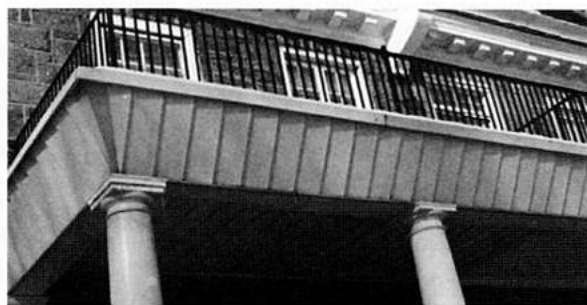
Aluminum cladding hides the original cornice details
